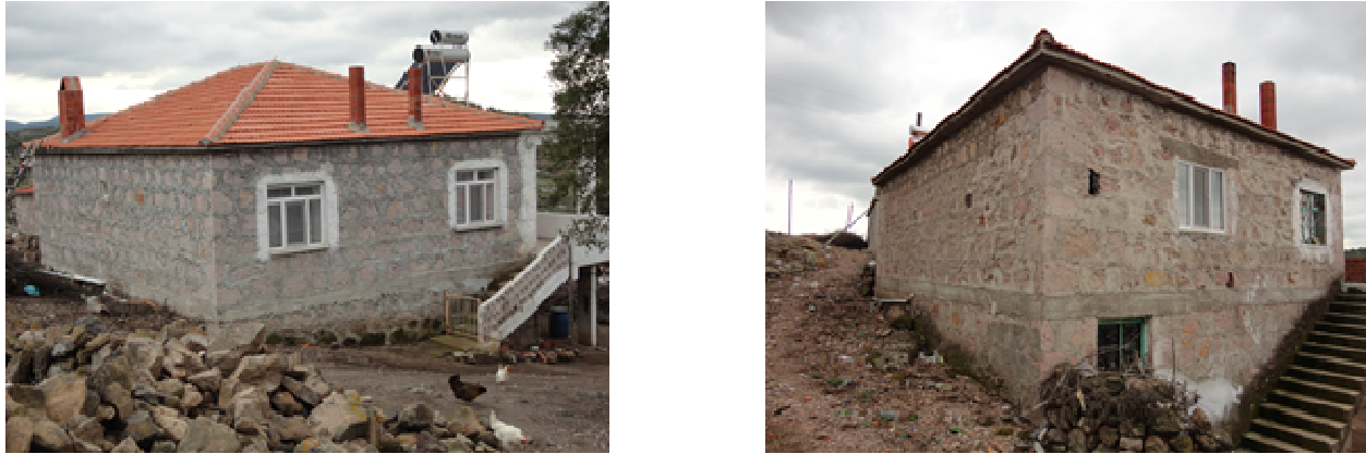
Figure 12. Examples of undamaged masonry structures
