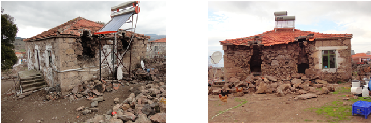
Figure 10. Examples of masonry buildings whose wall thickness was reduced during construction of fireplaces
