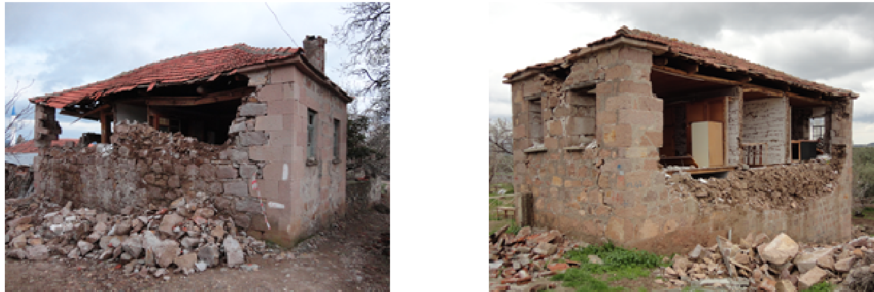
Figure 4. Examples of heavily damaged masonry buildings
